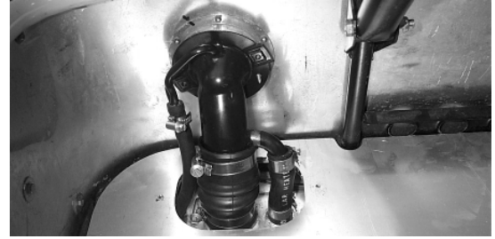
Fig 13 Filler cover and boot carpet removed
